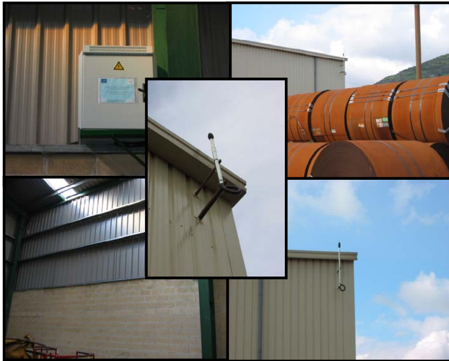
Figure #12: Mounting images of the FIX EQUIPMENT
