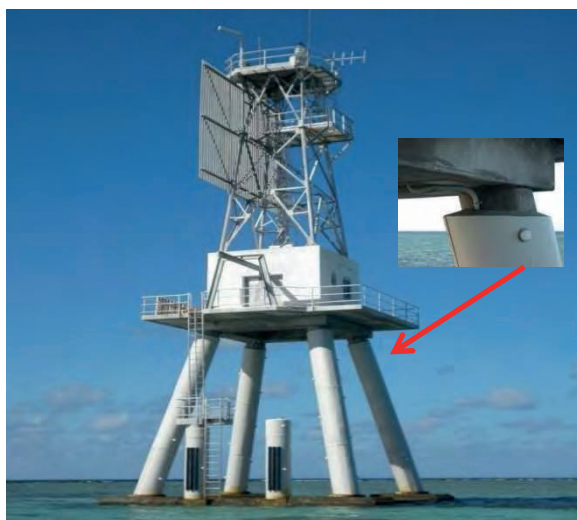
Figure 7: Hydrographers Passage structure with lifejacket fitted
